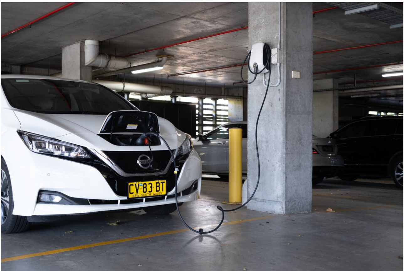
Charging point at the Goulburn Street parking station (Photo by Chris Southwood / City of Sydney)
